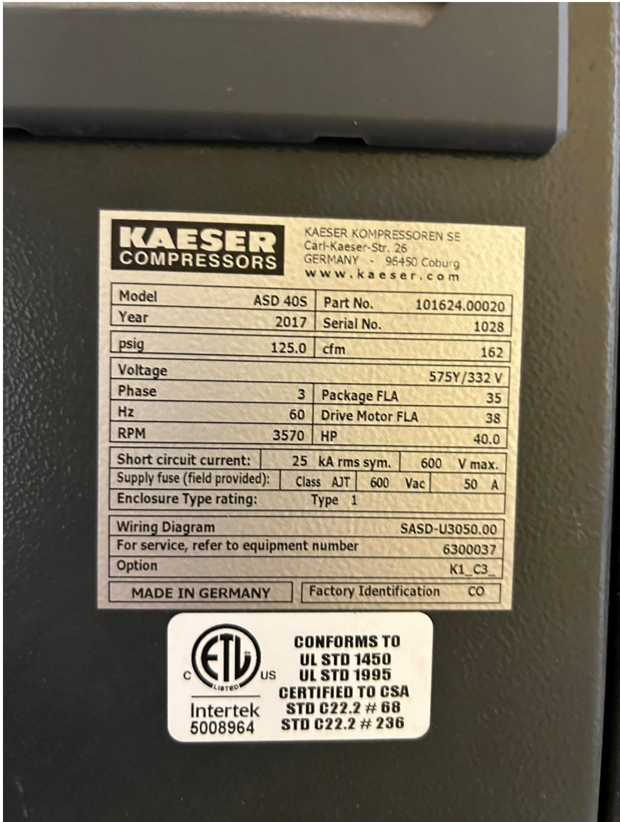
Fig 2.16 – Compressor name plate
