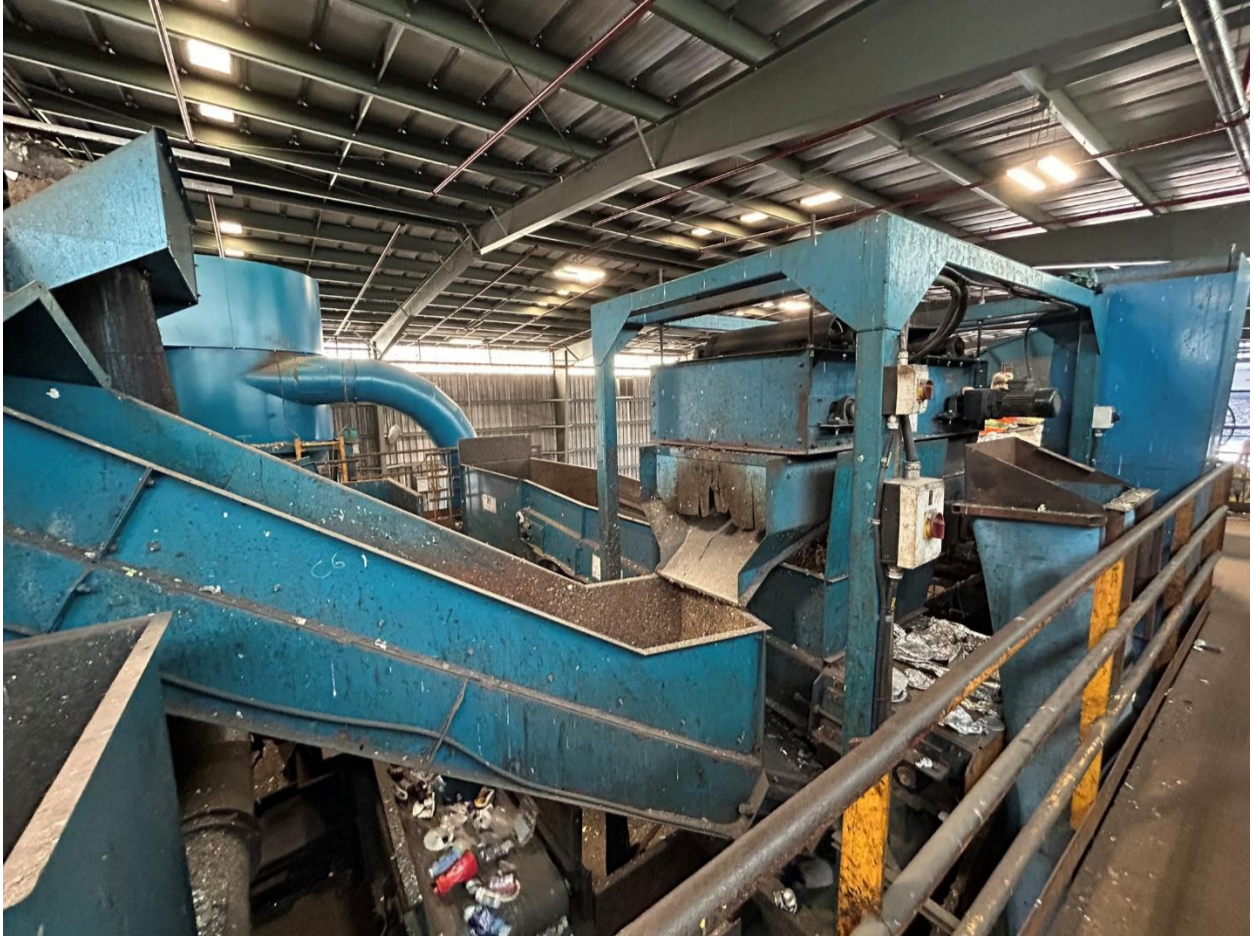
Fig 1.17 – Magnet conveyor located off cat walk
