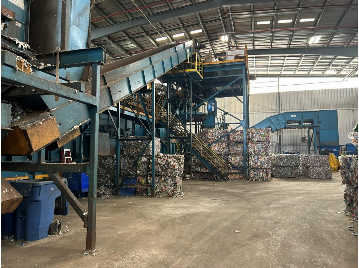
Fig 1.4- South portion of processing equipment and the baler infeed line
