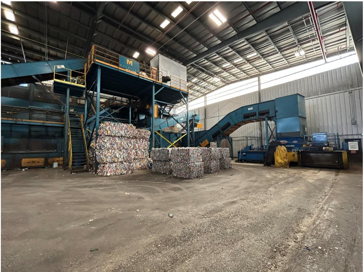
Fig 1.5- Processing mezzanine that houses the optic sorter and its compressor; along with baler
