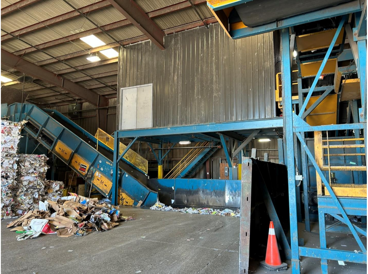
Fig 2.4- Compressor room and baler infeed underneath room
