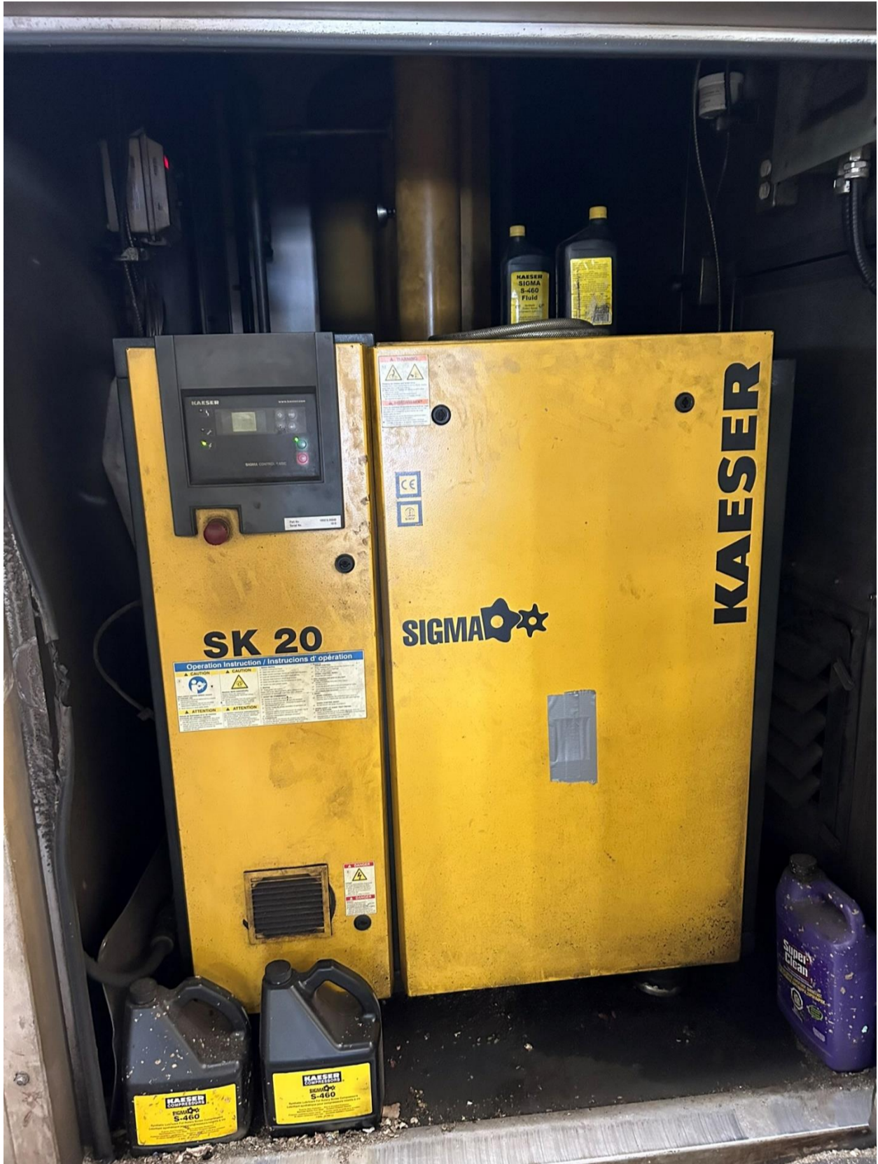
Fig 1.12 – Kaeser SK 20 located on the mezzanine next to the optic sorter that supplies the Optic system
