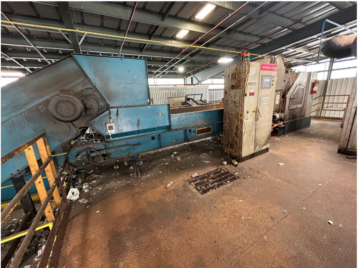
Fig 1.10 - Optic Sorter located on mezzanine
