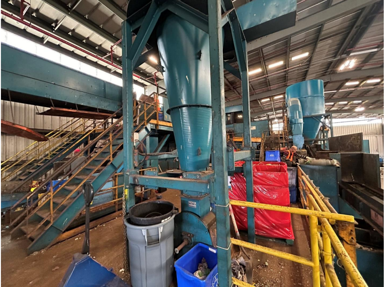
Fig 1.9 – Bottle processing area located up on mezzanine
