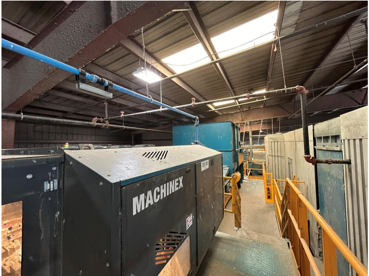
Fig 2.13 – Sort room sprinkler line disconnect point
