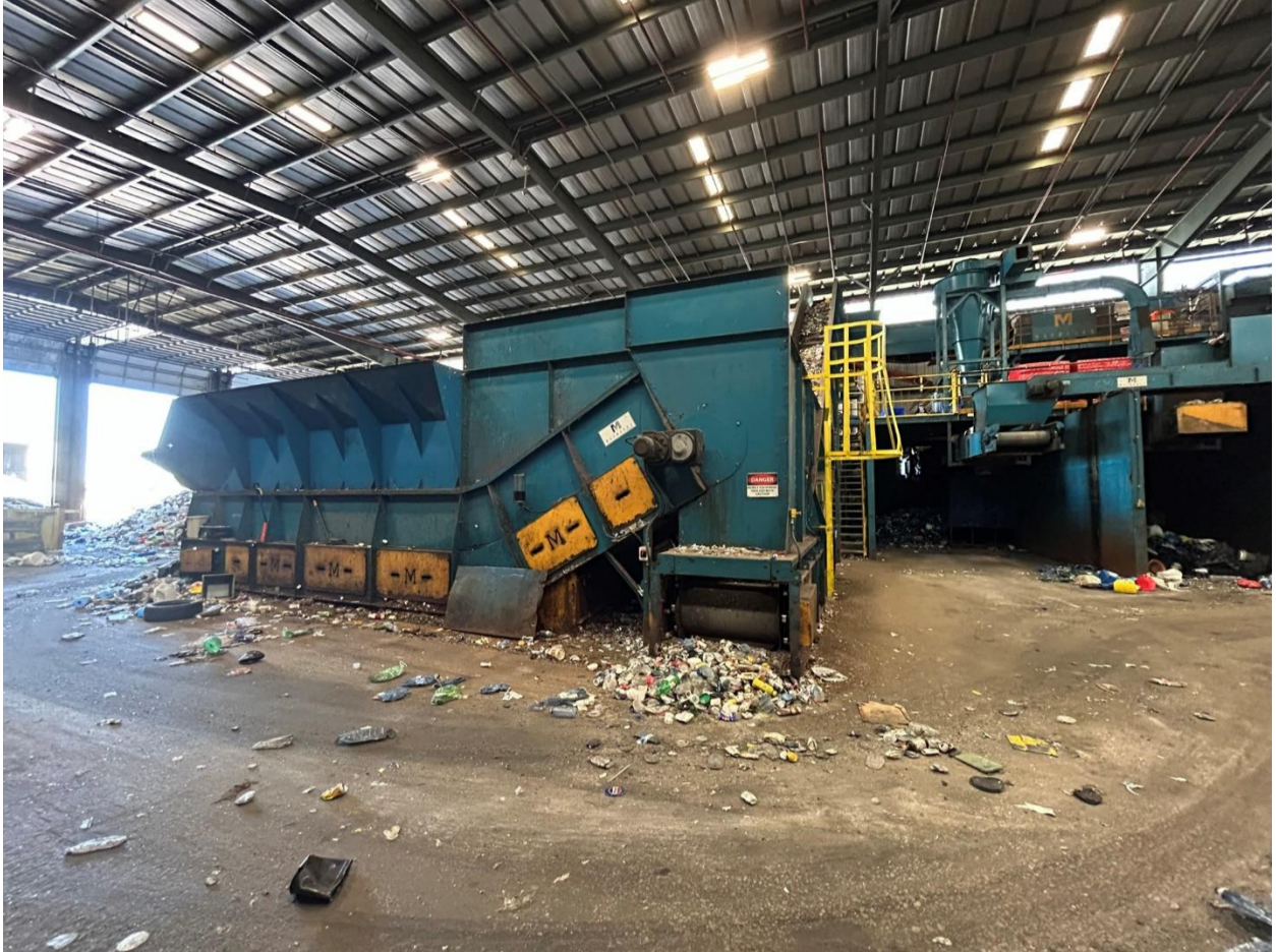
Fig 1.2 – South portion of C1 (hopper) feeds materials to the process line
