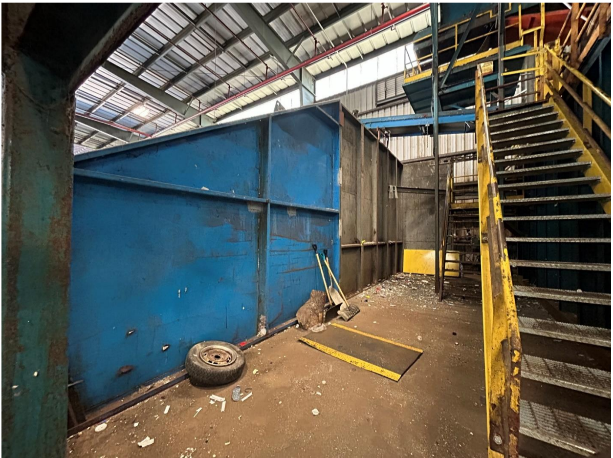
Fig 1.7- Push wall (NOT to be removed) adjacent to hopper that separates main processing equipment from tip floor.
