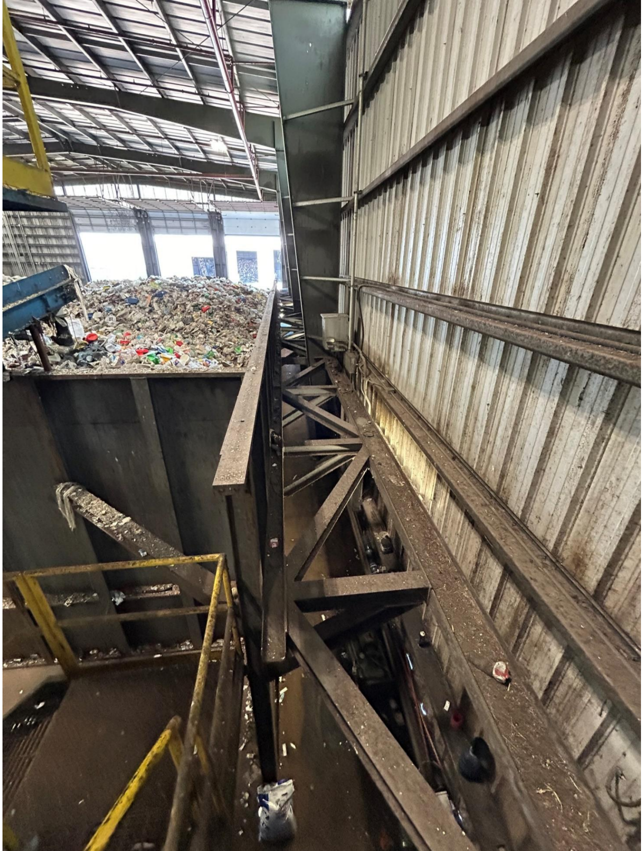
Fig 1.8 – Back of Push wall for the tip floor’s northeast side, along with supporting braces
