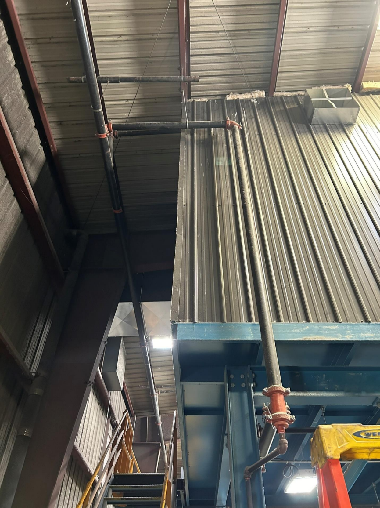
Fig 2.9 – Sprinkler line disconnect point (supply coverage under sorting equipment) on compressor sort room
