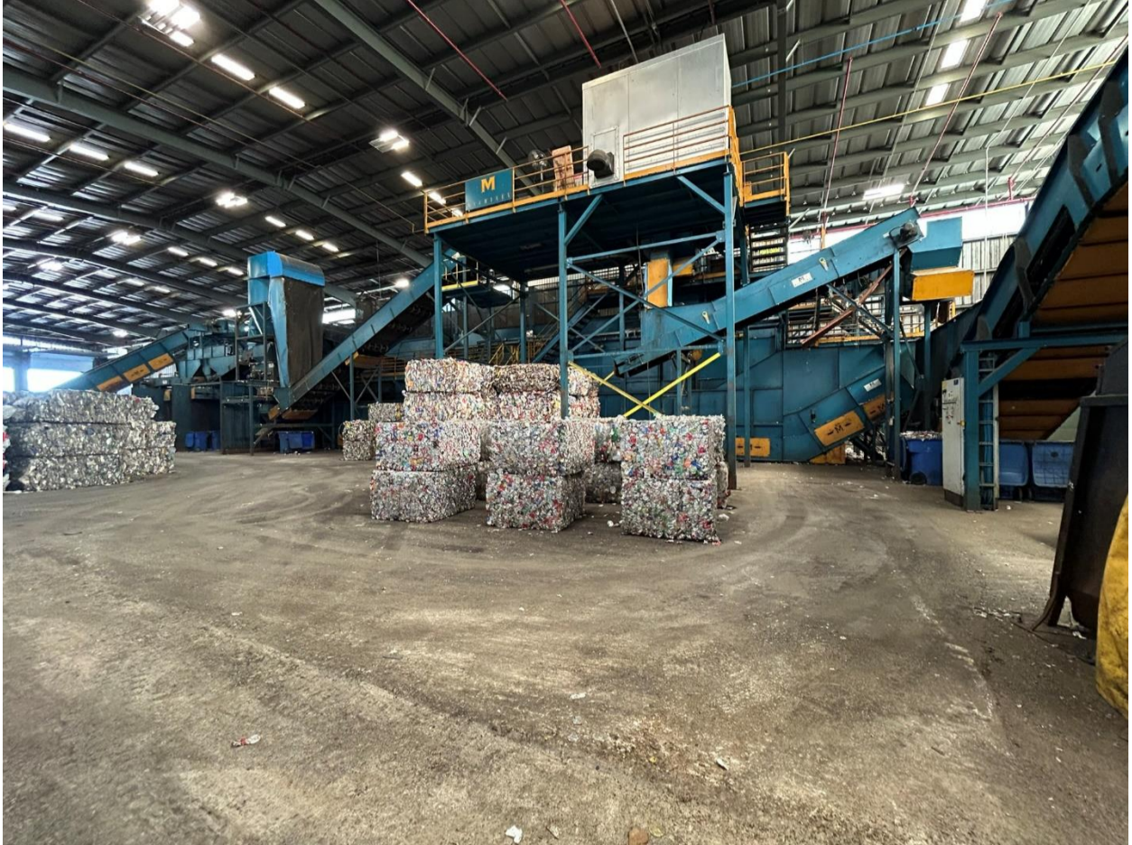
Fig 1.6 – Southeast view of process equipment, mezzanine and structure
