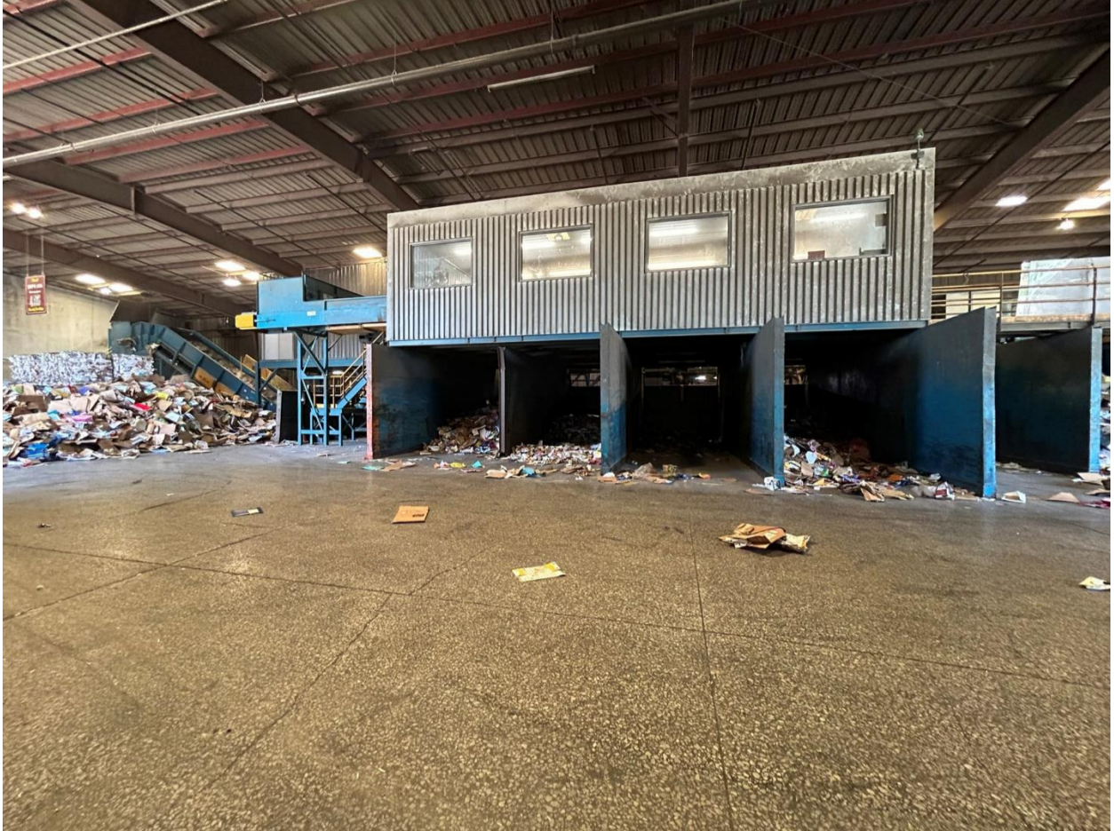
Fig 2.2- Processing equipment, bunker walls, and sort room
