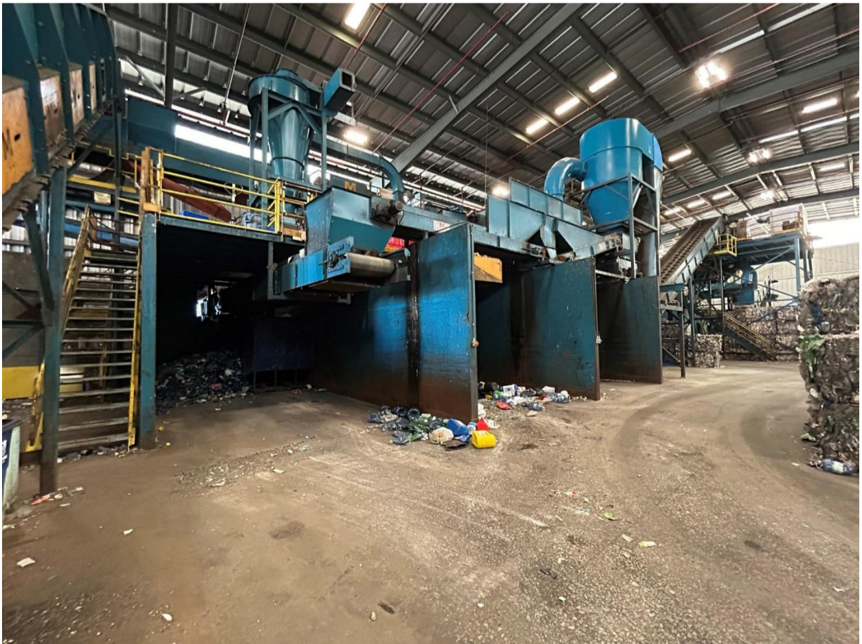
Fig 1.3- South portion of the processing equipment adjacent to C1 hopper
