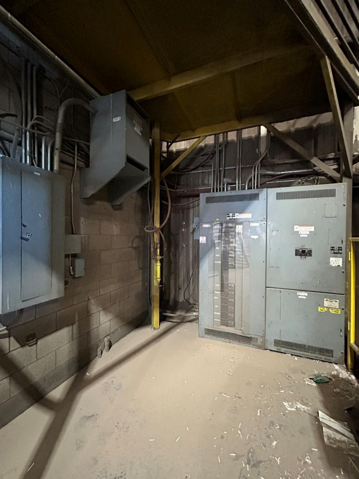
Fig 2.17 – Main distribution panel located on the west wall and south of baler
