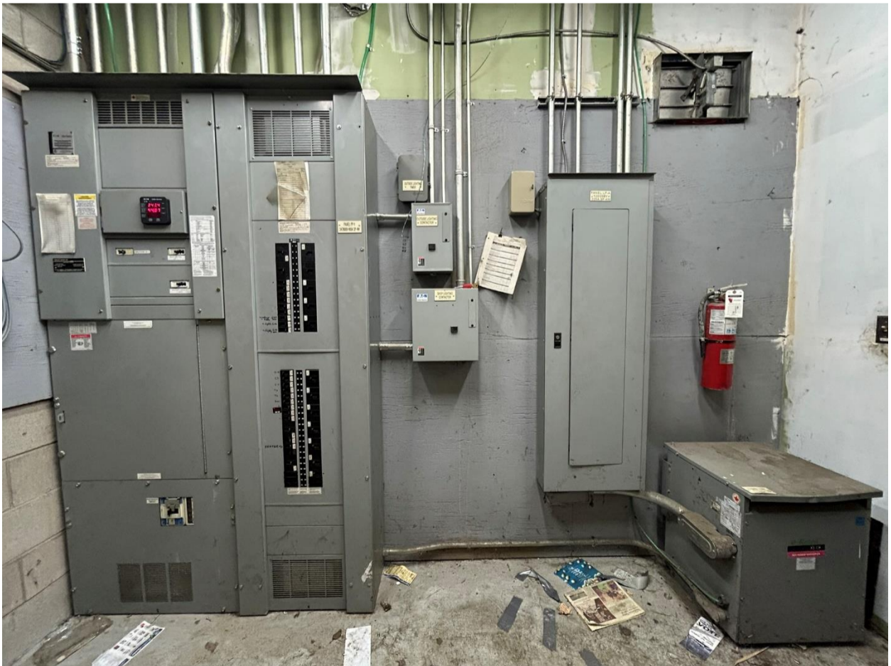
Fig 1.18 – Main Distribution Panels located inside panel room adjacent to lunchroom
